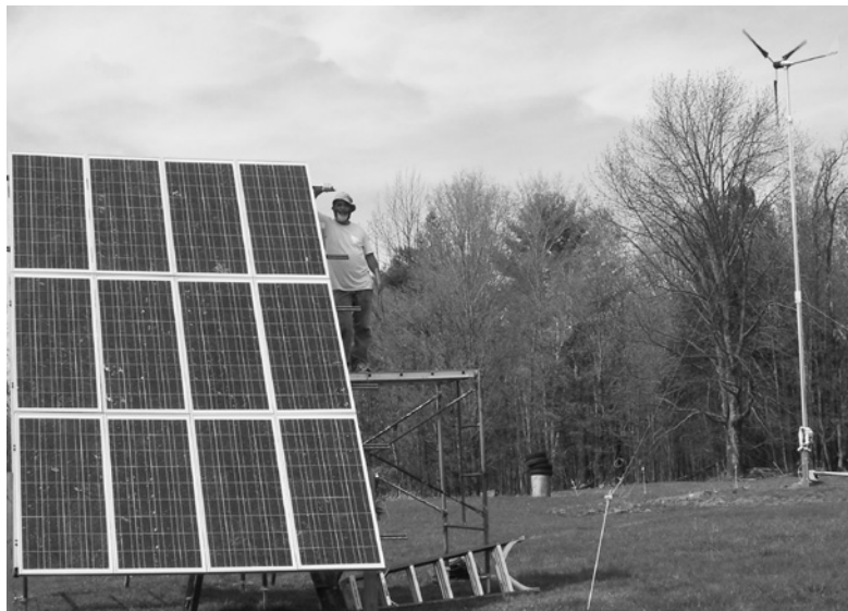
WEC member Ed Hutchinson stands proudly on a construction scaffold behind his 1.3- kW solar array. The power generated by this 12-panel array and the 1-kW wind turbine on the right goes to a battery bank in Ed and Alexandra Thayer's basement.
