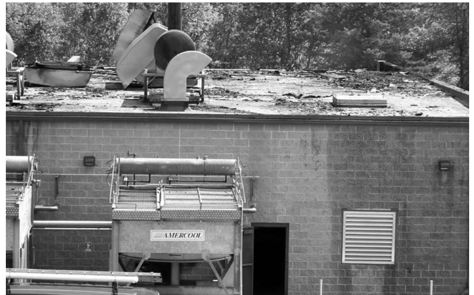
WEC's methane-powered generating station in Coventry suffered a fire on August 8. The fire was quickly contained, with damage largely confined to the roof and some of the equipment in the engine room.
