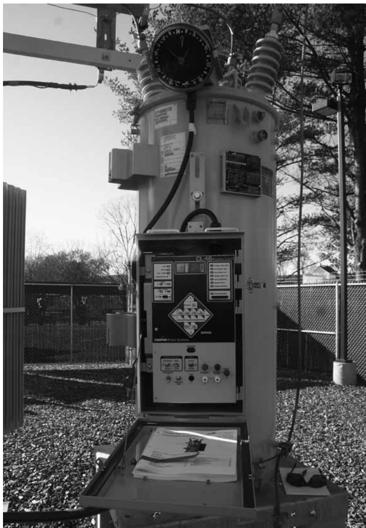
A new regulator at the East Montpelier substation. The voltage for each phase of the three-phase lines can now be more precisely regulated using the controls seen here (the box in normally kept closed).
