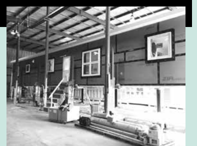
The VERMOD is a highly efficient, energy-saving alternative to the mobile home. Above, a unit nears completion at the factory in Wilder. For more on this project, and programs making it more affordable, turn to pages 4 and 5.
