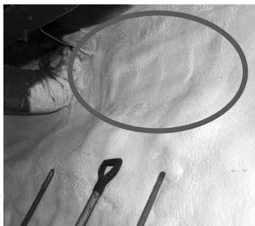
Ghost window! An important step for Bekah and Patrick was to have foam insulation sprayed in the basement of their old farmhouse. The frames of a now-covered cellar window can be seen above the shovel handle.
