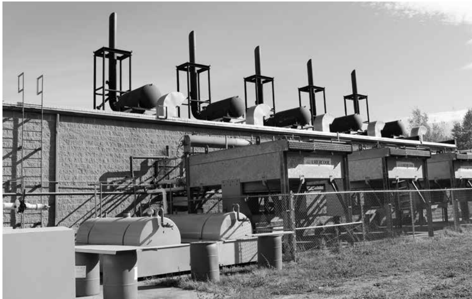
These five engines burn methane gas to create electricity that's roughly two-thirds of WEC's power portfolio. The engines are so hot that on a cloudless day, visitors to the plant could see heat shadows moving rapidly over the ground.
