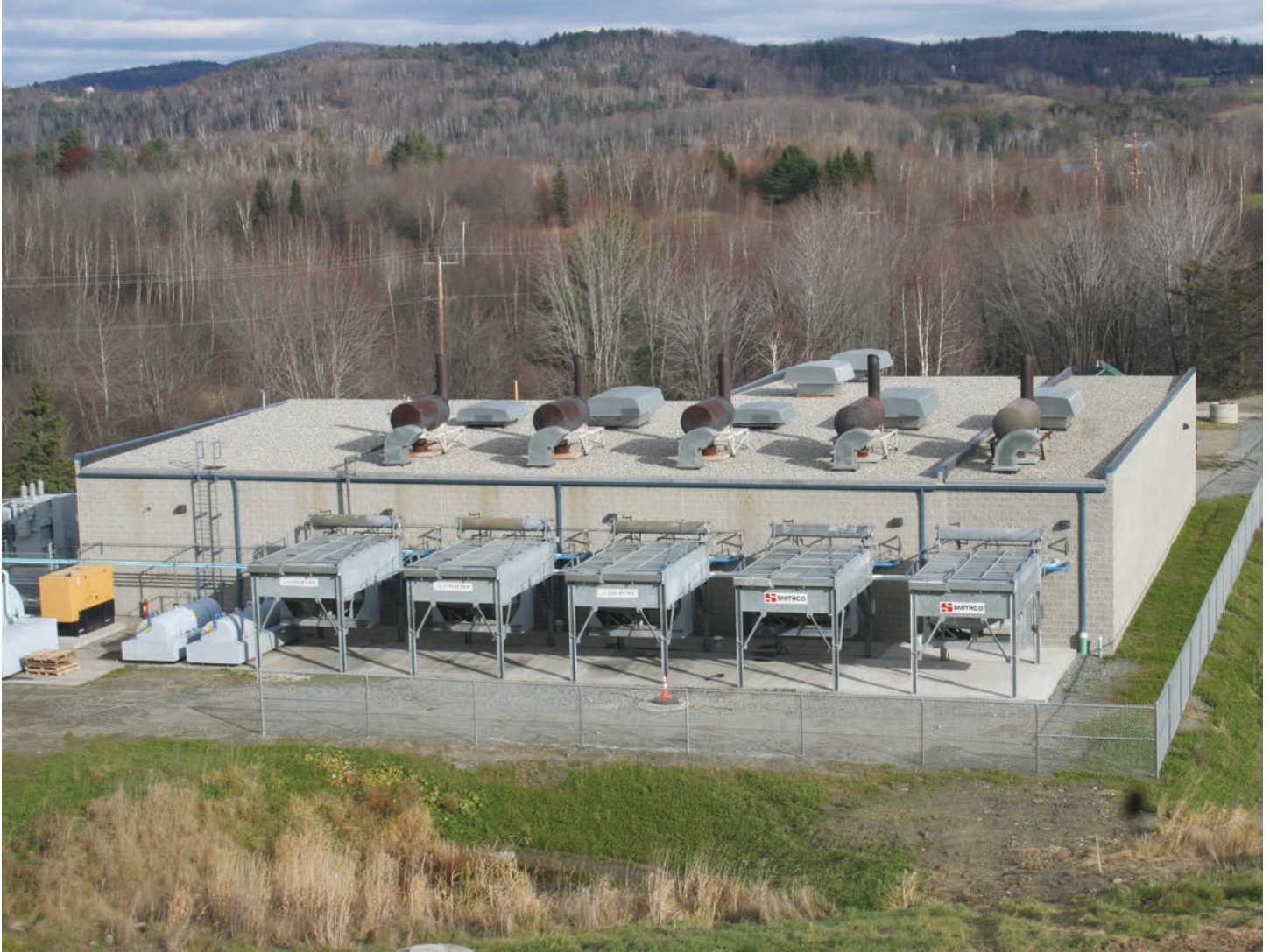
WEC's largest energy resource is the Coventry landfill gas to electricity plant. Increasing the number of generators at the plant will not only increase the energy generated but will help WEC with reducing peak demand due to electrification.
